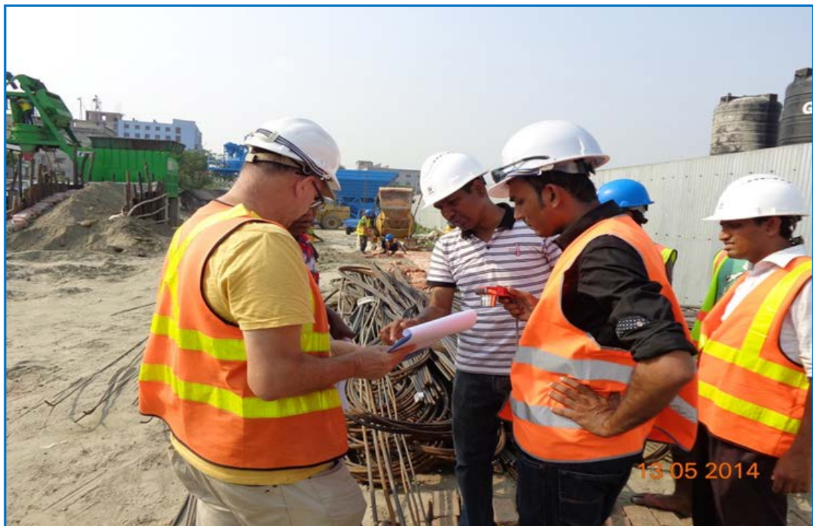
Shiddhirganj Power Plant Project – Client: Isolux-Corsan, Spain Civil Works of Power Plant
